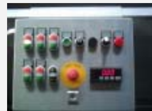
The control panel
